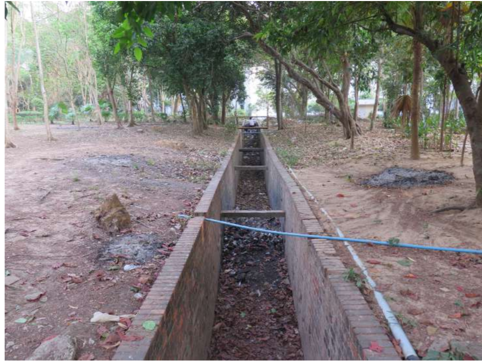
Typical drainage channel with debris and rubbish building up at its base
